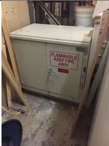
Flammable locker in tool room.
