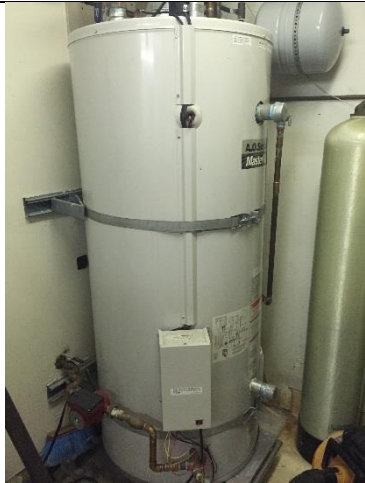
Site water heat in kitchen closet.
