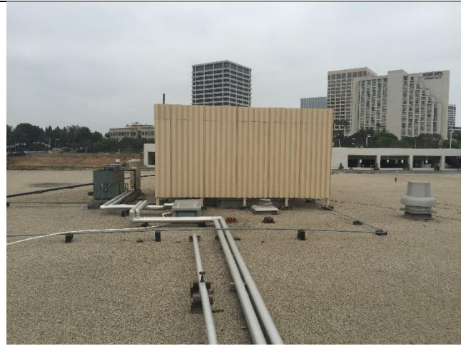
Roof top HVAC system housing.
