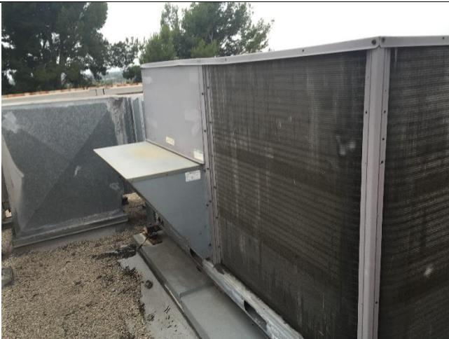
Add-on HVAC system on roof top.
