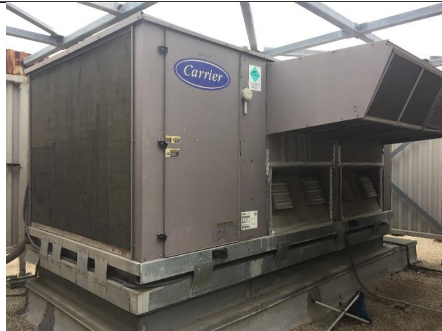
HVAC system on roof top.
