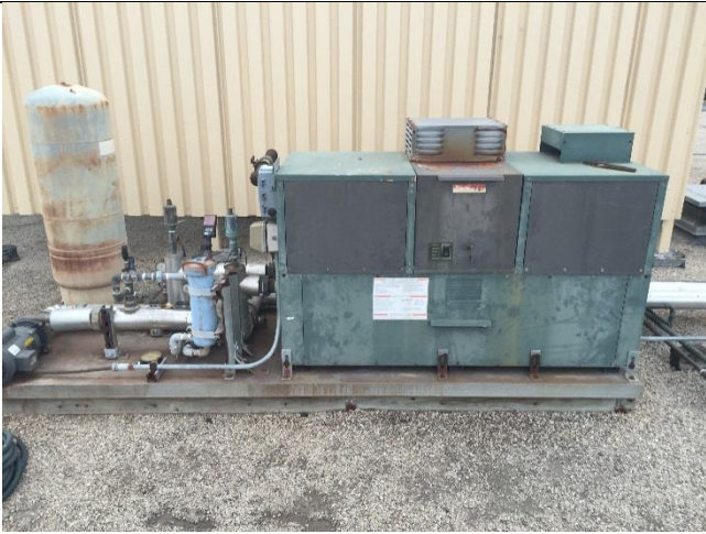
Roof top boiler.
