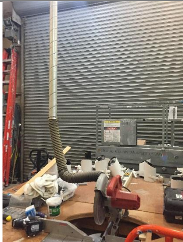
Tool shop dust collection on tools.
