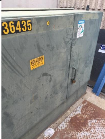
Incoming site power source.
